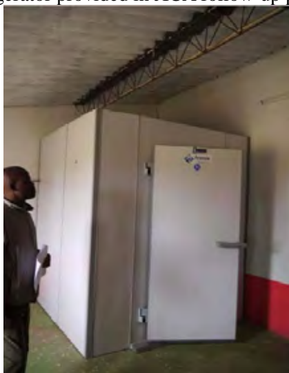
Refrigerator provided in JICA follow-up project
