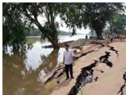
Riverine collapsed at the Night Market, Panchor in April 2008
