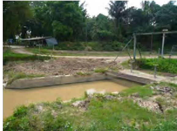
There are a number of water intake points along the Muar River. This picture shows the pumping station at Kpg. Jambu Lapan, Negeri Sembilan.
