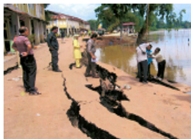
River bank collapsed at the Night Market, Panchor on April, 2008
