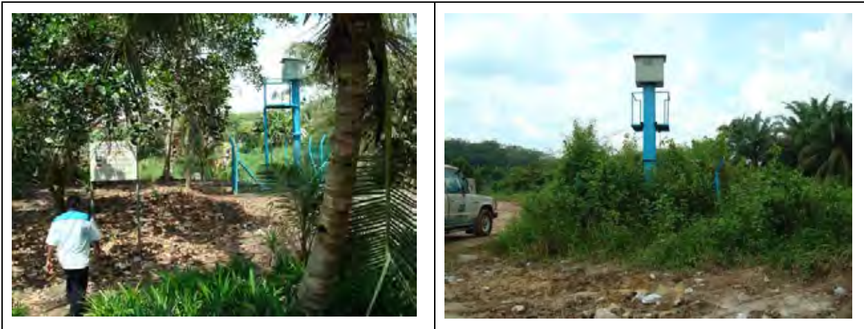
Figure 8.2.3 Flood Warning Siren (Kg. Tiong and Taman Sg. Gemas)
