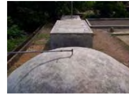
Digester, anaerobic baffled reactor (ABR) and anaerobic
