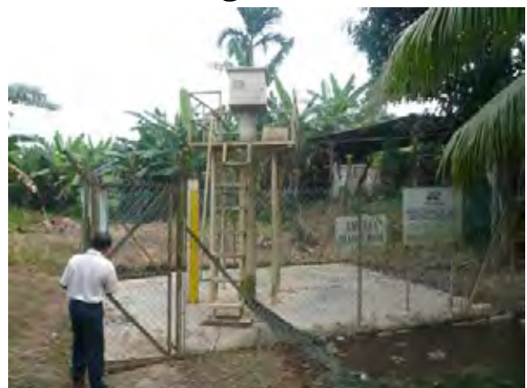
The existing flood warning siren at Kpg. Chedong, Maran.
