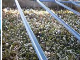
Ecological trickling filter
