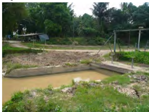
There are a number of water intake points along the Muar River. This picture shows the pumping station at Kpg. Jambu Lapan, Negeri Sembilan.
