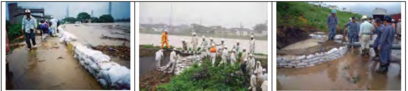
出典: Flood Fighting in Japan, Ministry of Land, Infrastructure, Transport and Tourism of Japan
