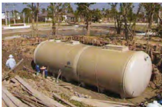
Figure 5.4.1 Sewerage Treatment Facility
