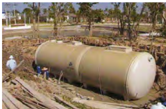
Figure 5.4.1 Sewerage Treatment Facility
