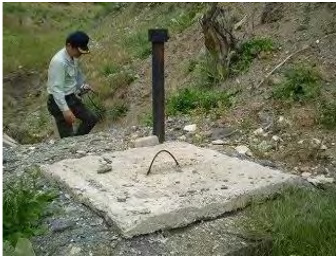
Photo 8 Water tank in the riverbed
