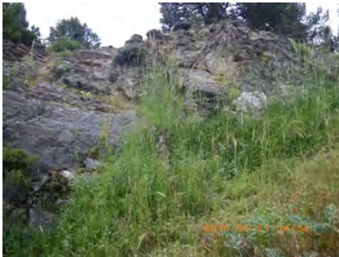
Photo 5 Lime which were dissolved and transferred along joints were deposited on the surface of the outcrop at the dam site
