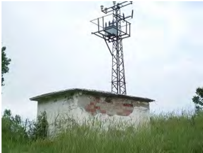
Photo 5 Water-pumping facility at the upper dam site
