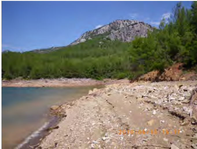
Cohesive soil washed out from clay stone by wave along the lakeside Photo 8 Tailrace and Outlet site
