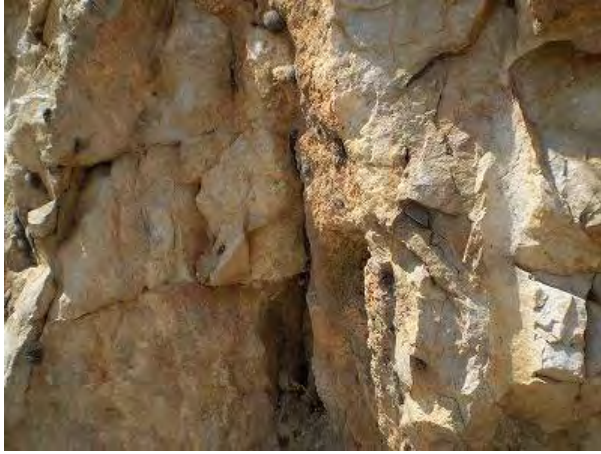
Photo-11 Cavern along Cracks in Limestone
