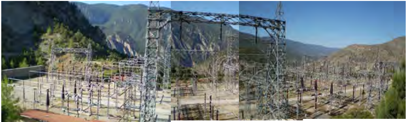
Photo 5.48 Existing Switch yard (Upstream Left Bank of Dam)
