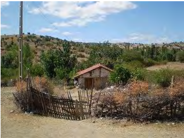
Photo 5.45 Affected Storage House
