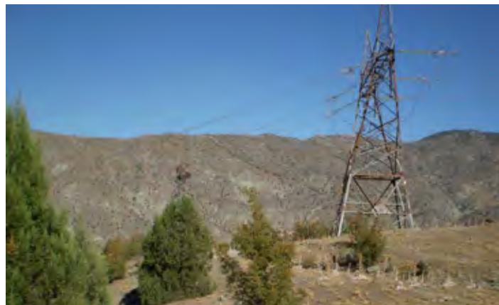
Photo 5.49 Transmission Lines from Existing S.Y to Upstream (2 Systems)
