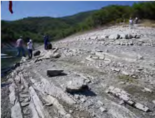
Photo 5.12 Weathered, turned edges of the mudstone which is bending to the south due to creep
