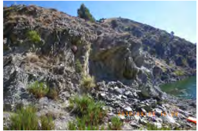
Photo 5.29 Loosened rock on the surface of creeping rockmass at the outlet site
