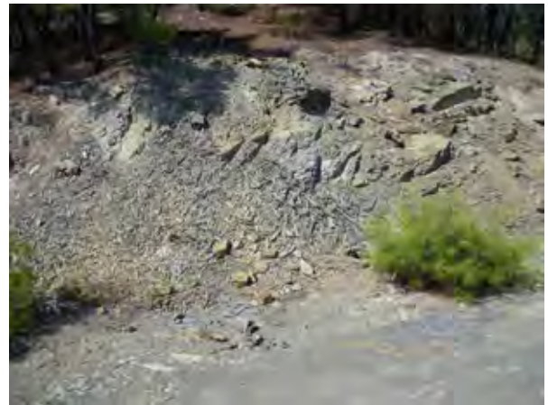
Photo 5.13 Crumbling and disintegrated mudstone due to slaking
