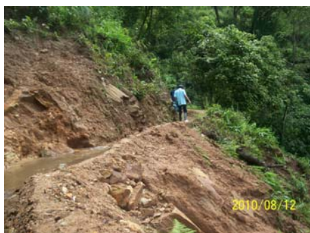
Destructed Canal Caused by Floods
