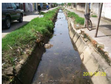
Deformation of Main Canal and Disposal of Solid Waste
