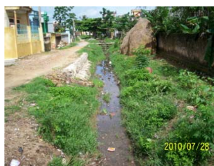
Deformation of Secondary Canal and Disposal of Solid Waste
