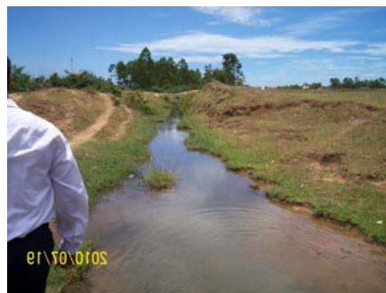
Deformation of North Main Canal
