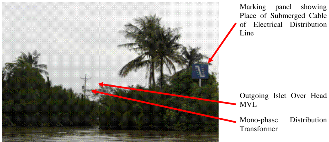
Figure 4.1-8 Submerged Medium Voltage Feeder Cable (Ben Tre Province, Ke Sach District)
