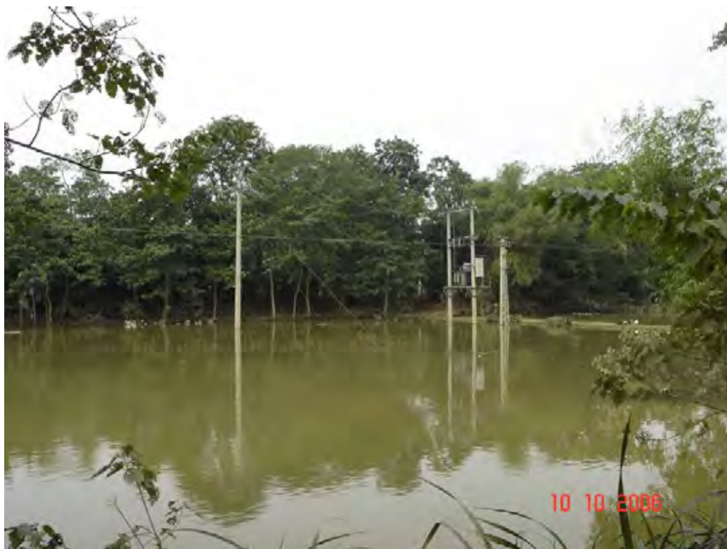
Figure 4.3-1 Damaged Electricity Facilities (Ha Tinh Province, Huong Son District, Son Think Communes)
