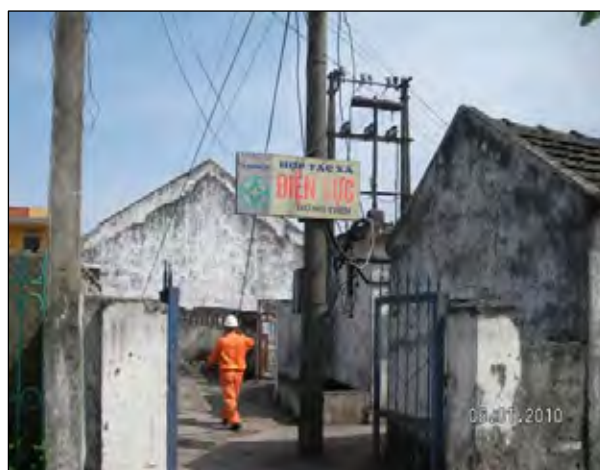
Figure 5.1-1 Maintenance Conducted by Kim Son Electricity (District Electricity) of Low Voltage Facilities which belongs to Hung Tien Power Supply Cooperative (Ninh Binh Province, Kim Son District)
