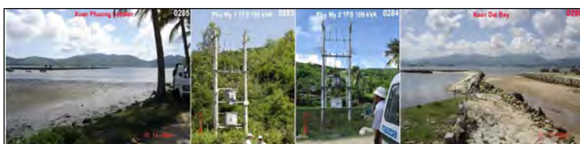
Figure 6.2-16 Lobster Breeding Beach in Xuan Phuong Commune, SPL Phu My No.1 and Phu My No.2 Distribution Transformer (Power Source for Sea-Product Area), Lobster Breeding Zone in Xuan Dai Bay
