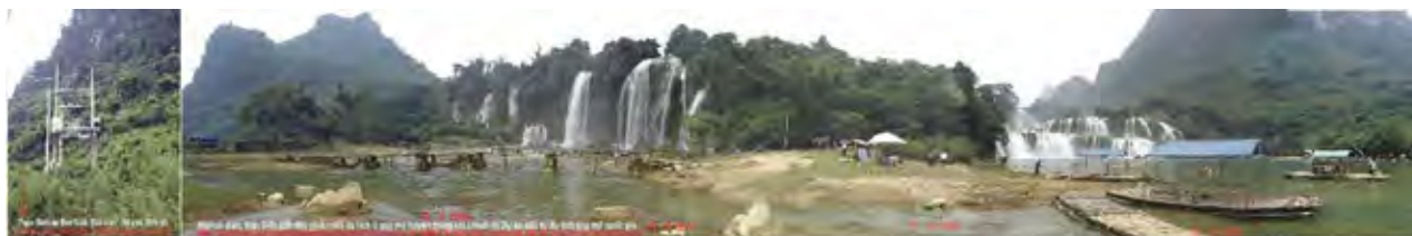
Figure 6.2-8 Ban Gioc Waterfall with its Distribution Transformer (50 kVA) Installed under SPL III
