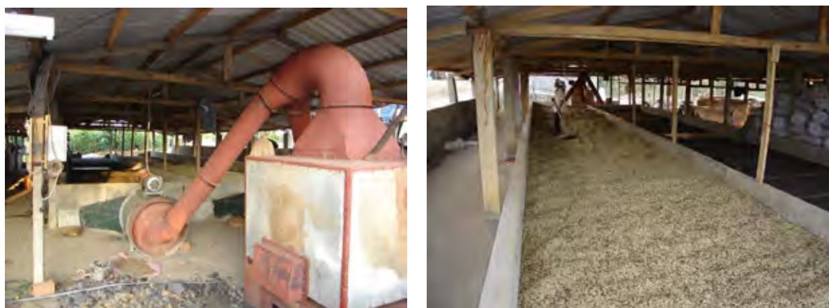
Figure 6.2-3 Electric Ventilator, Coffee Kernel Dryer - Conveyor
