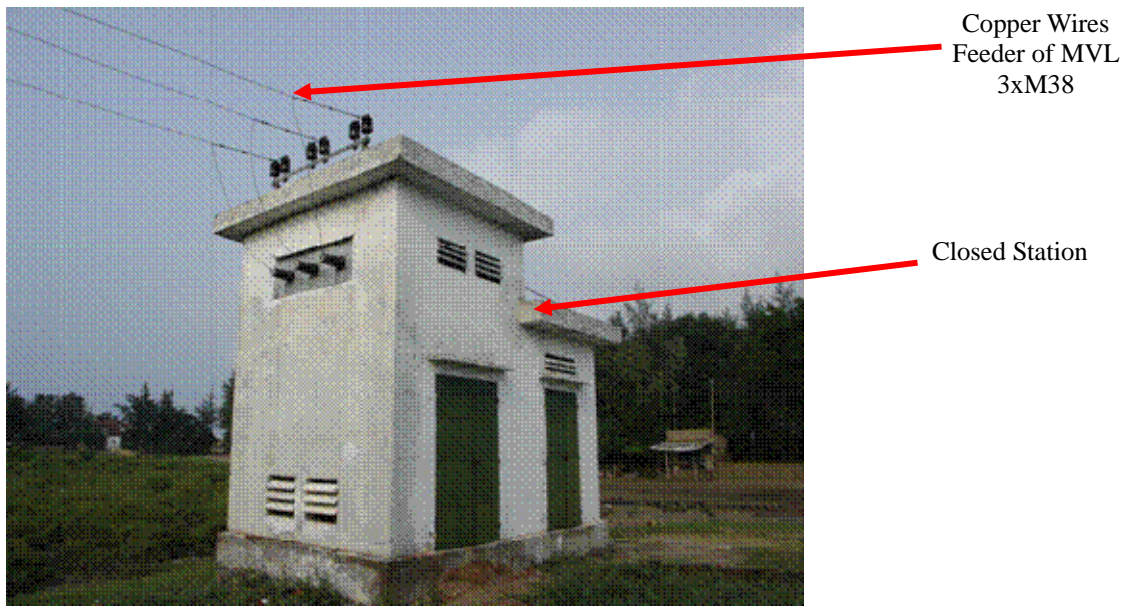
Figure 4.1-7 Cam Nhung Commune Electric Line of Cam Xuyen Coastal District in Ha Tinh Province
