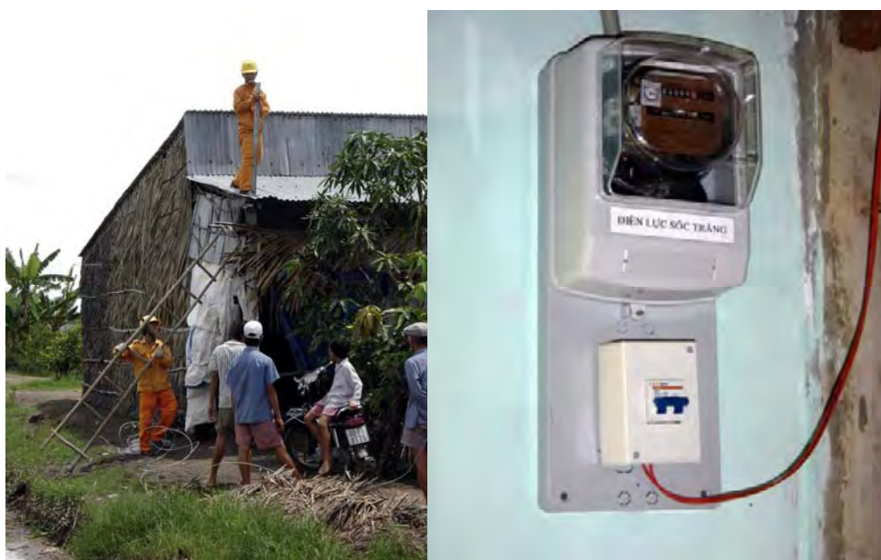
Figure 4.1-6 Electricity Workmen Implementing the Drop Service for Inhabitants' Household in Thanh Phu Commune of My Xuyen District in Soc Trang Province
