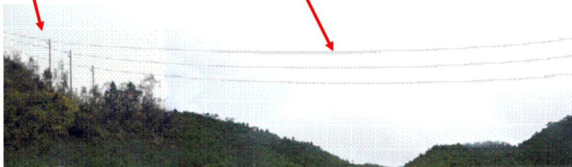
Figure 4.1-10 Long Span Medium Voltage Line (Tuyen Quang Province, Yen Son District)
