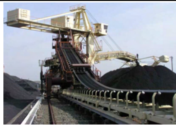
Stacker 2,000t/h Max piling height 9m
