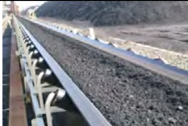
Belt conveyer (receive) 1,550t/h, Length 1.3km
