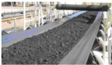
Belt conveyer (deliver) 2,400t/h, Length 900m
