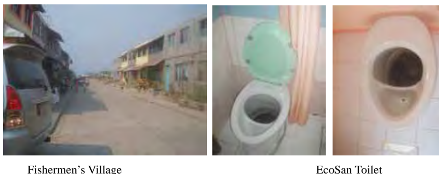
Figure D. 3.3.3 EcoSan toilet in the fishermen's village in San Fernando City in La Union Province
