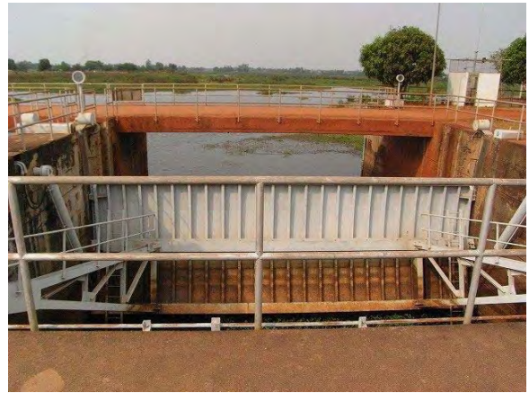
Gate of Barrage (Radial Gate)
