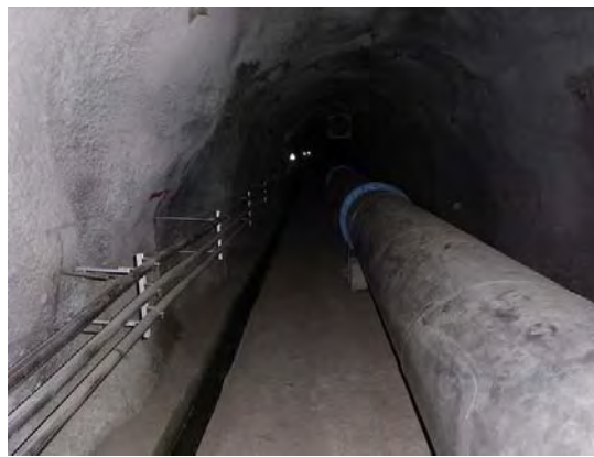
Water Diversion Pipeline in the Tunnel from Huai Pai Reservoir
