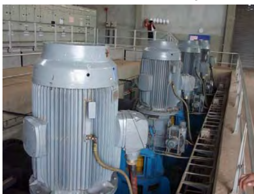
Fig. 1 Head Regulating Pumps ( 2.3\text{m}^3/\text{s} \times 4\text{units} )
