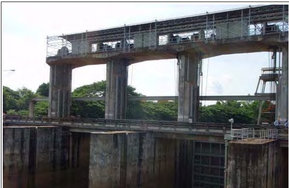
Huai Luang Estuary Barrage located in Udon Thani Province. It was constructed at the river mouth of Huai Luang, which is one of tributaries of Mekong River. Main functions of the barrage are to prevent back water from Mekong River in rainy season and to store discharge from Huai Luang in dry season. Watershed area and whole length of Huai Luang is 4,340km 2 and 100km,
