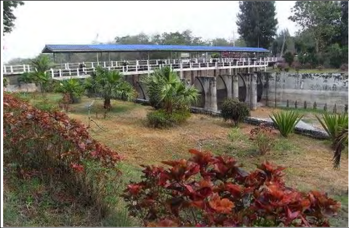
Lam Takhong Dam spillway in Nakhon Ratchasima Province. It has radial gates.
