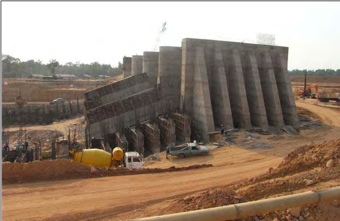
Construction of Lam Pao Dam spillway in Kalasin Province. It has 4 radial gates, their height and width are 7.70m and 12.5m, respectively. The maximum discharge of this spill way is 2,216\text{m}^3/\text{s} .
