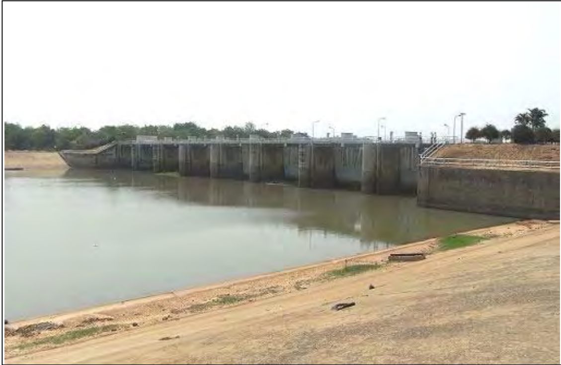
Yasothon Weir in Yasothon Province, which irrigates 9,760ha. This photo shows the scene from upper right bank.
