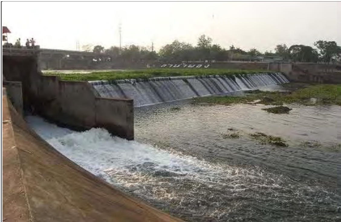
Nong Wai weir in Khong Kaen Province. It was constructed to irrigate 48,320ha farmland in Khong Kaen Province and Maha Sarakham Province.
