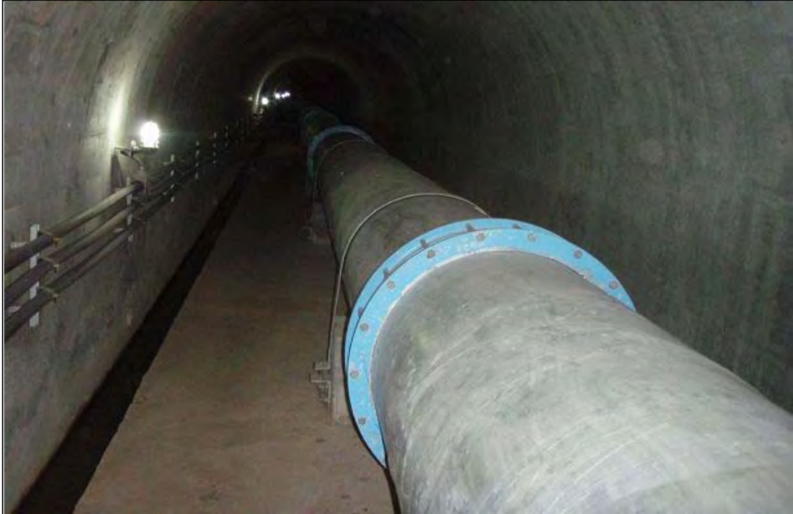
Pipeline inside of the 710m-length tunnel (diameter 3m) from Huai Phai reservoir in Mukdahan Province. The diameter of this pipeline is 1.2 to 0.8m. This is one of components of water diversion project, namely, Lam Phayang Pumipat Project. It is possible to divert 6MCM water to Huai Phai irrigation area (12,000ha) in Kalasin Province.
