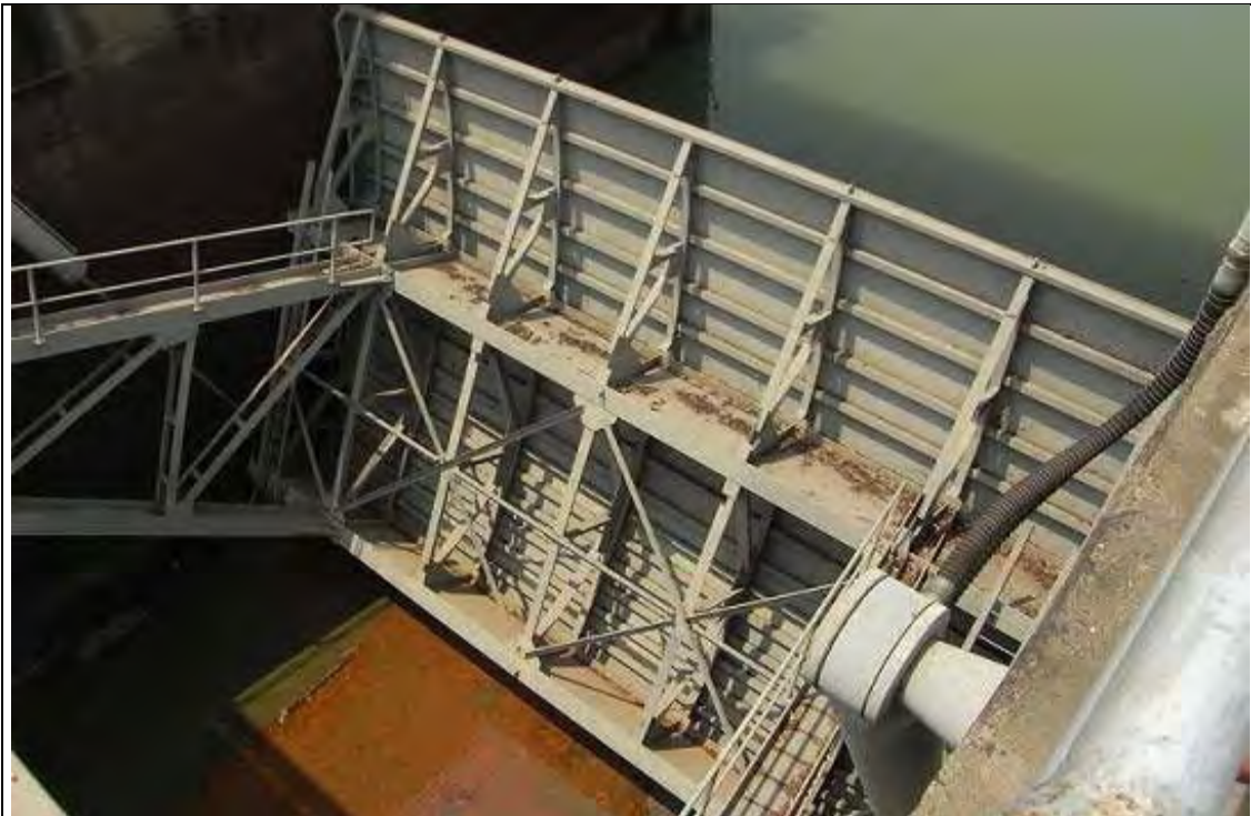
Rasi Salai weir in Sisaket Province, which irrigates 5,500ha farmland. Timing of gate opening is decided based on the gate operation committee consisting of farmers in upper and down stream, RID, TAO staff. The gate is opened for around 4 months period per year.
