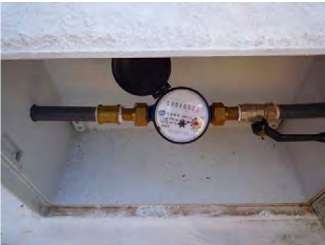
Tap water measurement meter
