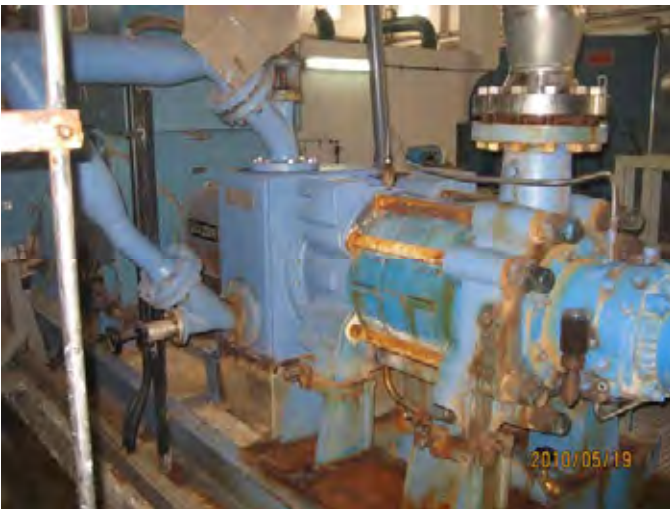
High pressure pump with energy recovery device (Praia)
