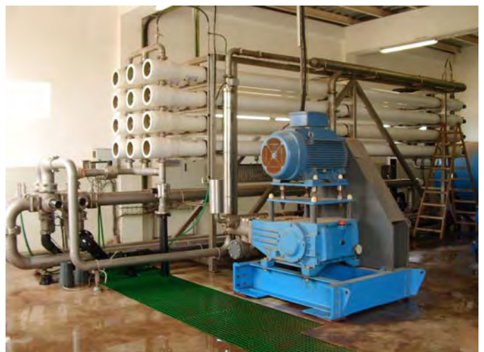
High pressure pump with energy recovery device (Sal island)
