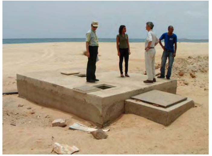
Intake beach well (Sal island)
