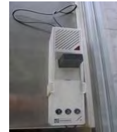
Toll Booth Intercom
