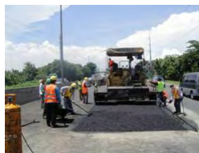
Deep Patch Repair Area
