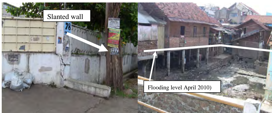
Photo 3.1 Sample of Subsidence Phenomena in Dayeuh Kolot
