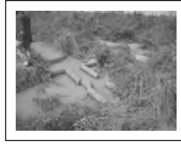
Iron plate gate at hand of tertiary box
