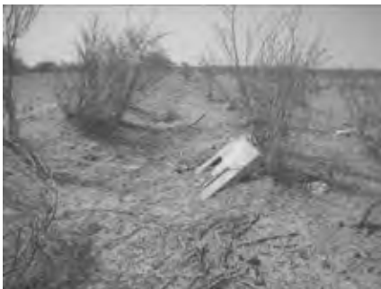
Quaternary canal diversion facility (Removal of sediment, banking and gate of iron plate are necessary)
