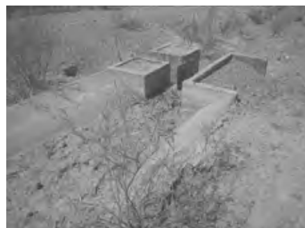
Secondary terminal canal diversion facility (Module Amasuk)
