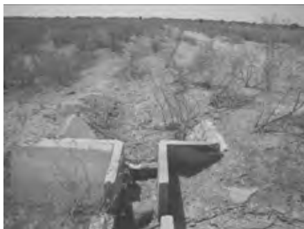
Diversion facility to tertiary canal
