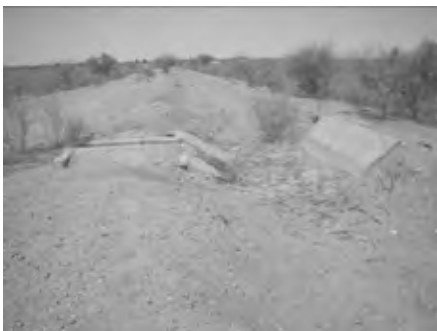
Secondary canal diversion facility
