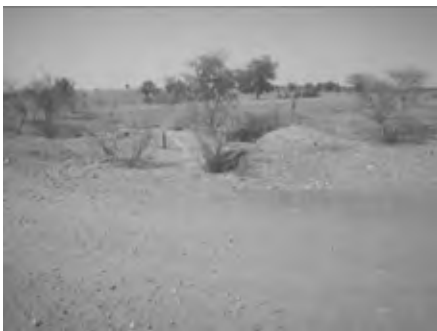
Diversion check gate
