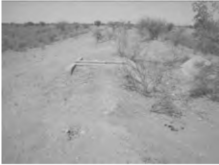
Secondary canal diversion facility
