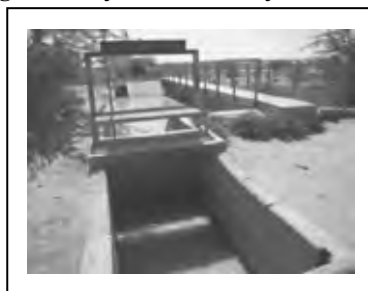
P2 Primary canal S27 Diversion facility
