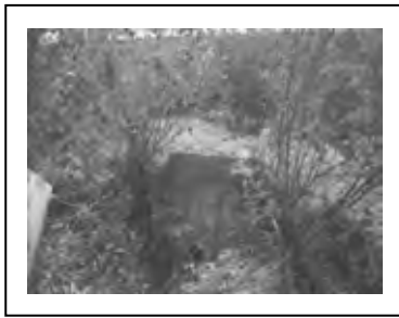
Intake water pipe from tertiary to fourth canal
