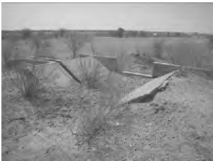
Diversion check gate
