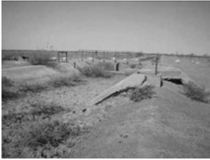
S9 Primary canal diversion gate and spillway (Right bank)
