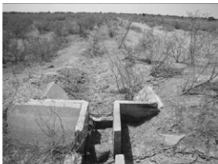
Diversion facility to tertiary canal
