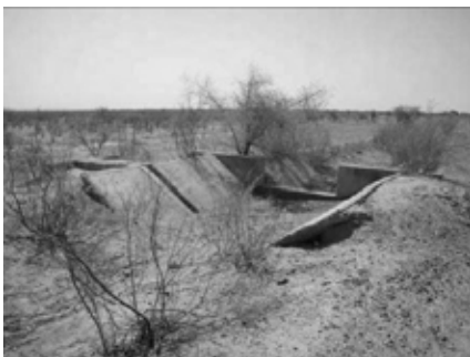
Drop and diversion regulating gate
