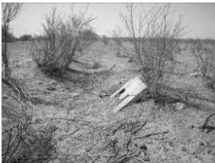
Quaternary canal diversion facility (Removal of sediment, banking and gate of iron plate are necessary)
