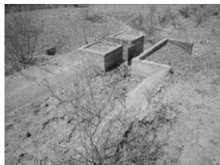
Secondary terminal canal diversion facility (Module Amasuk)
