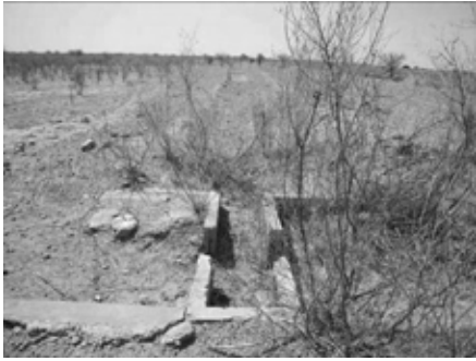
Tertiary canal diversion box
