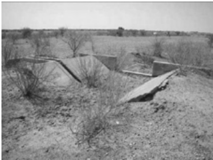
Diversion check gate
