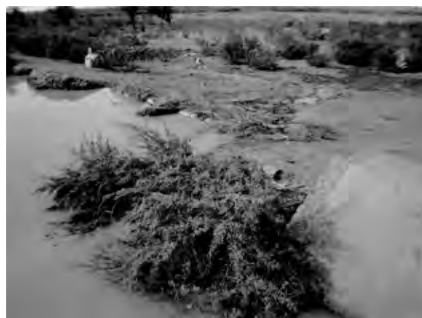
Damaged primary canal (P1)
