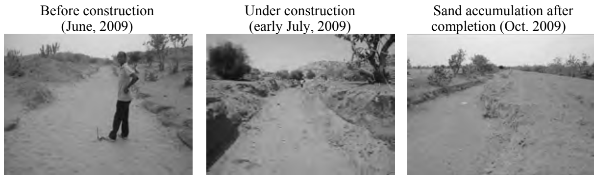
Excavation of Drainage Canal on the Left Bank of OA Primary Canal
