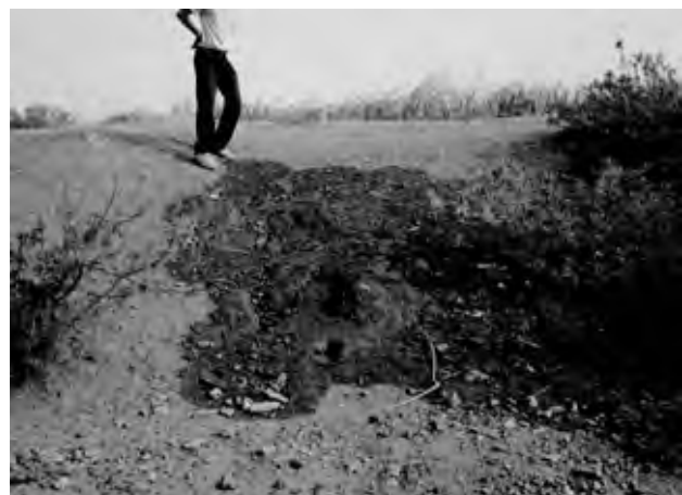
Before reinforcement of dike with sandbags Humid part of dike in downstream of SF7
