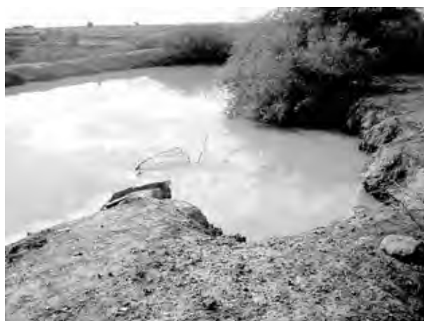
Damaged primary canal (P2)
