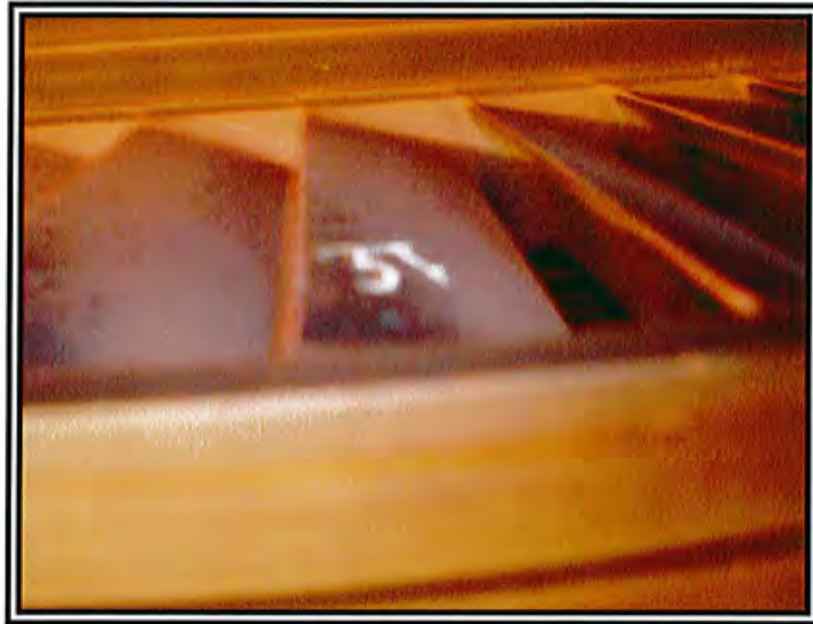
Photo 3 IP Rotating Blade – Surface Roughness of 3 rd Stage
