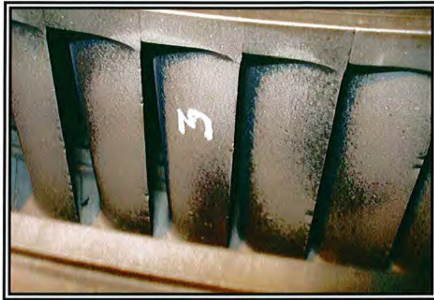
Photo 3 IP Rotating Blade – Surface Roughness of 3 rd Stage
