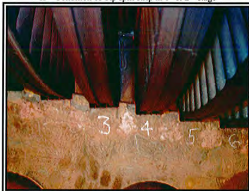
Photo 16 IP –Condition of Tip spill strip in 3 rd , 4 th , 5 th stage
