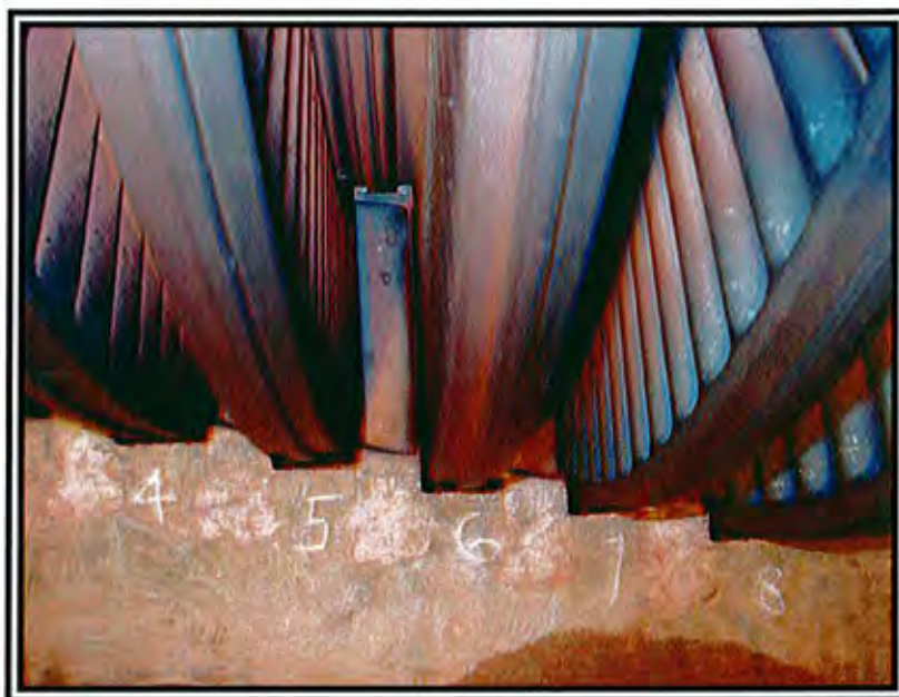
Photo 17 IP –Condition of Tip spill strip in 4 th , 5 th , 6 th & 7 th stage
