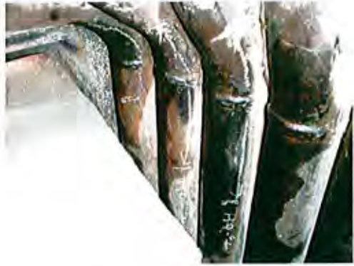
Erosion part at 1 corner
