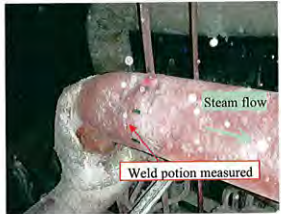
Measurement point of left De-superheater pipe
