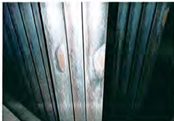
Erosion of Platen SH tube at the highest level of soot blower [extracted from Table II -18]
