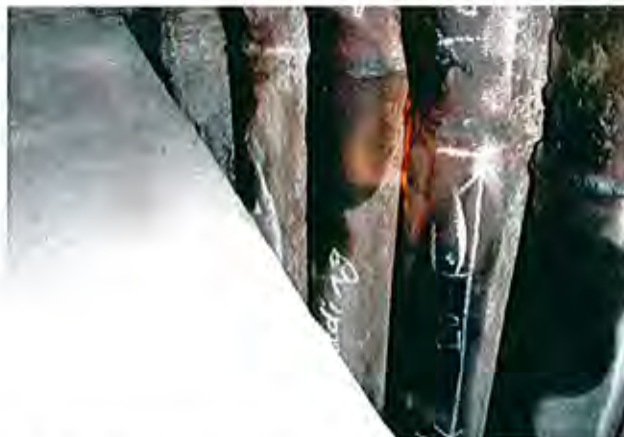
Erosion of Water Wall tube around burner portion [extracted from Table II -12]
