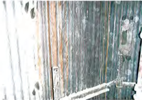
Erosion of Water Wall tube around corner portion [extracted from Table II -12]
