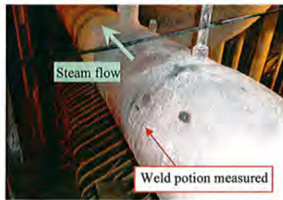
Measurement point of left De-superheater pipe
