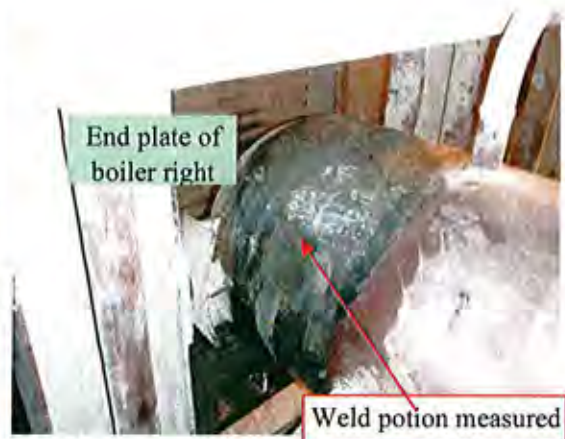
Measurement point of right RH outlet header
