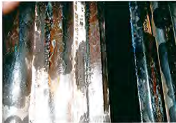
Erosion of front wall tube [extracted from Table I -12]
