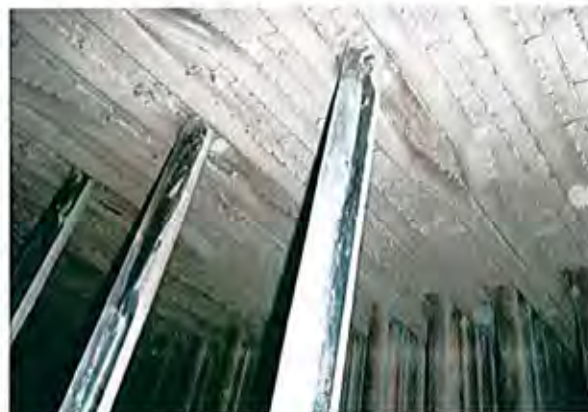
Erosion of rear wall screen tubes [extracted Table I -12]
