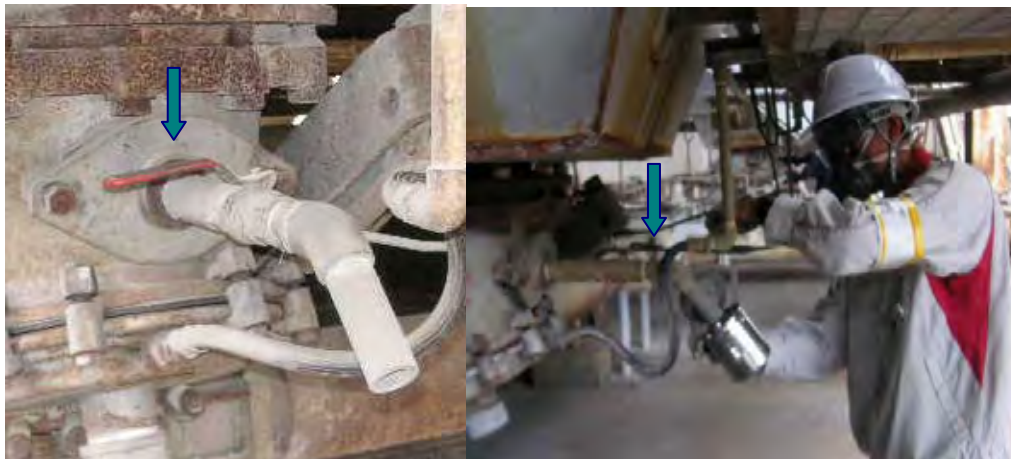
Fig. 6.13-2 Fly Ash Extraction Valve for Sampling
