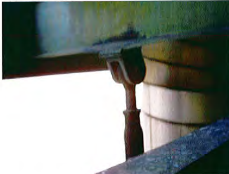
PHOTO 1- Bent supporting flange of I-beam at Y-restraint
