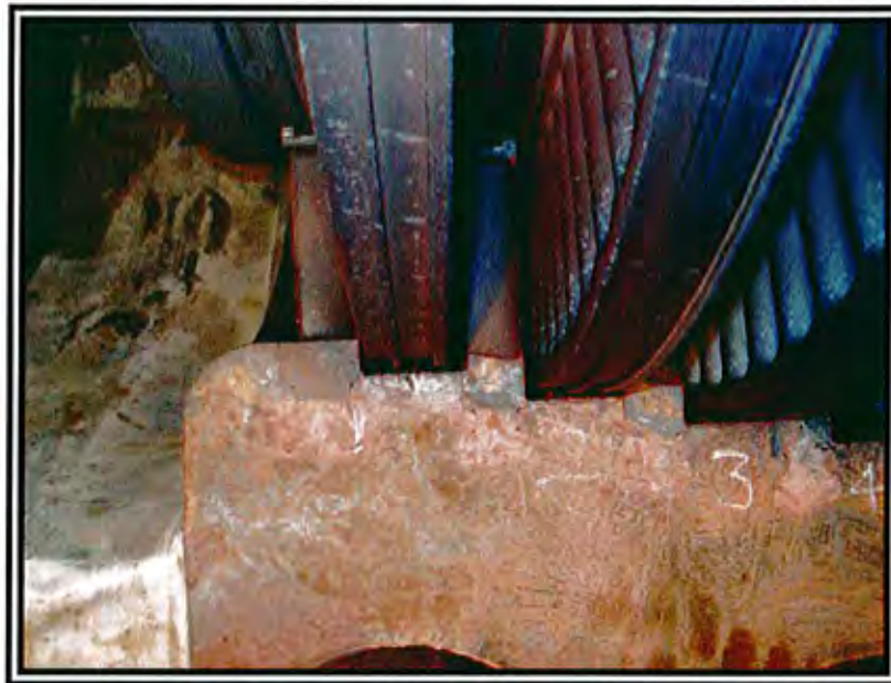
Photo 15 IP –Condition of Tip spill strip in 1 st & 2 nd stage
