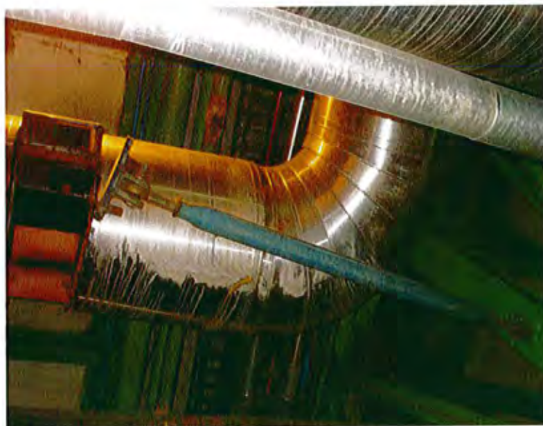
PHOTO 2- Dismantled Horz restraint in LPBP piping
