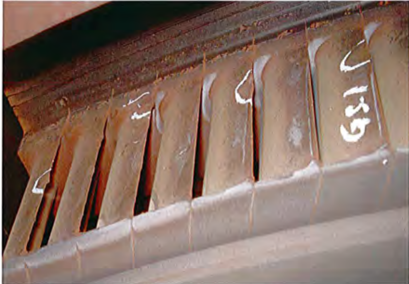
The view of damage of fixed blade profile of LP top outer casing
