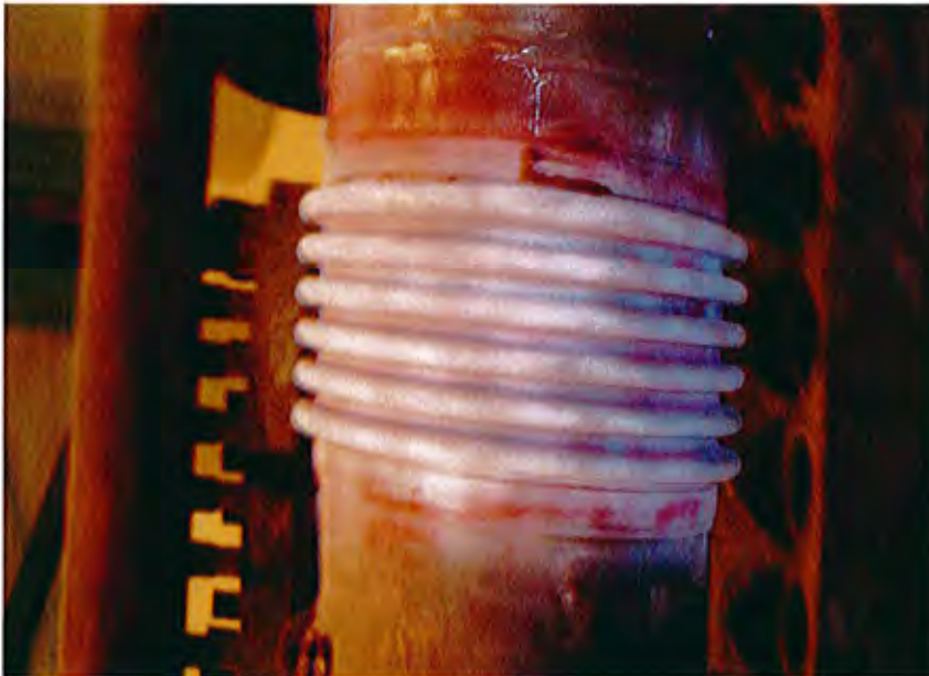
The LPT on expansion bellow of IP top outer casing
