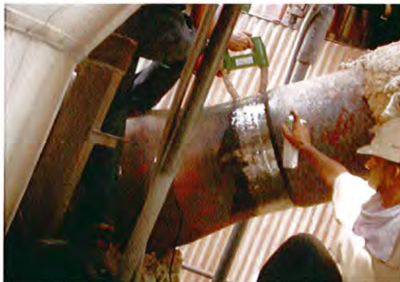
The view of MPI testing on Y joint of MS line 6 th floor.
