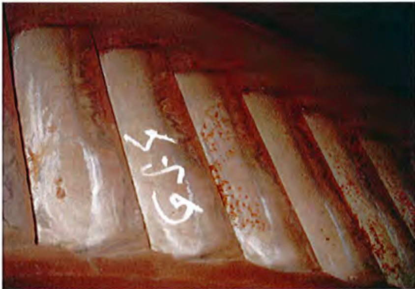
The view of deposits on LP top outer casing diaphragm blades.
