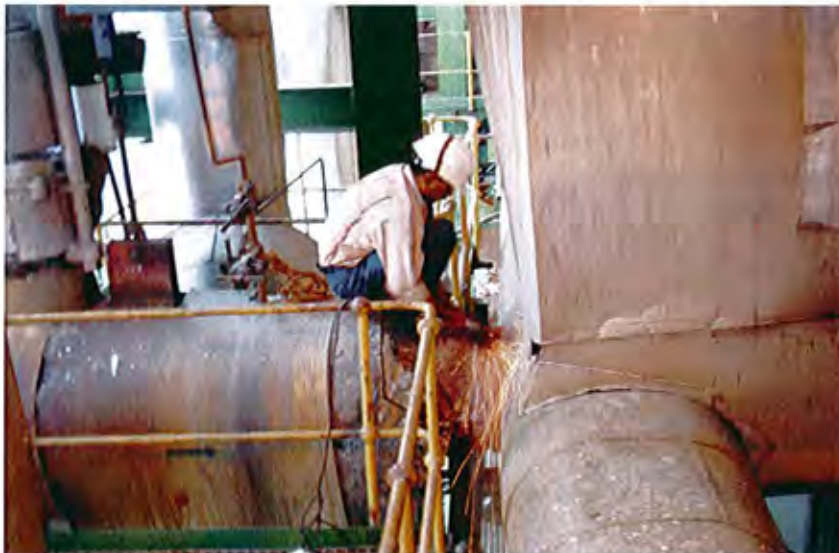
The cleaning of weld joint for testing at CRH line 9 th floor.
