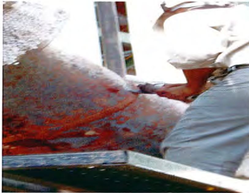
The view of weld joint cleaning at Y joint of HRH line.
