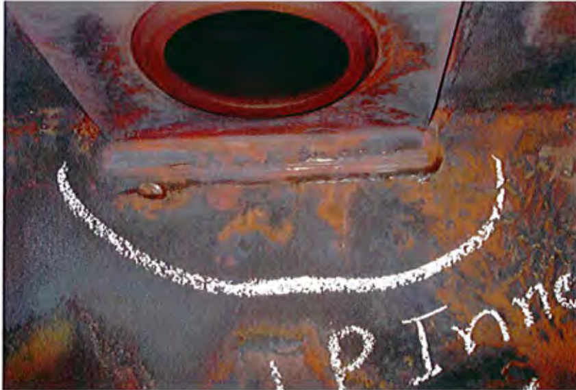
The view of erosion on LP top outer casing.
