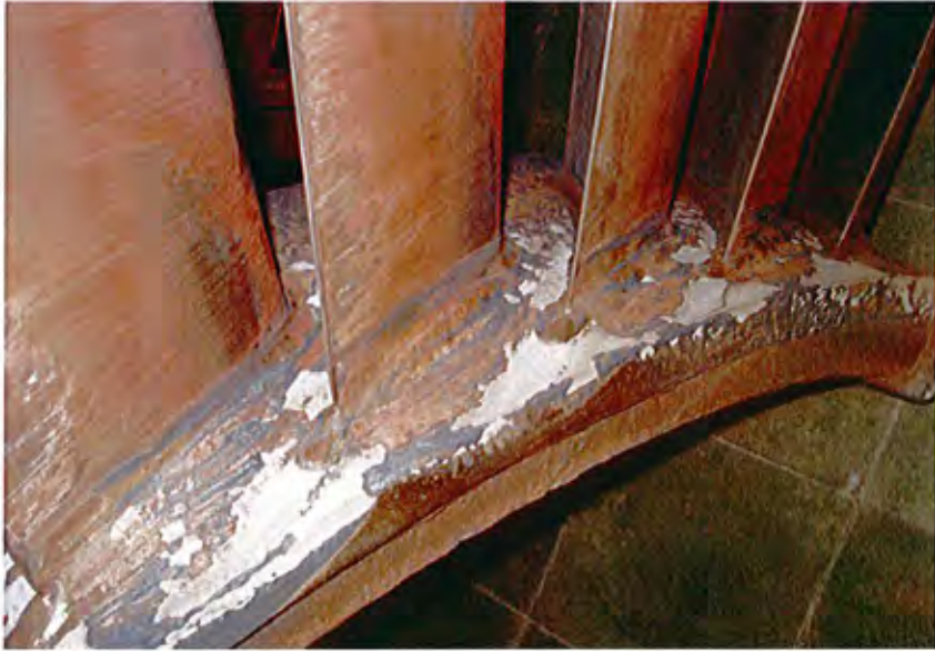
The view of deposits on LP top outer casing.
