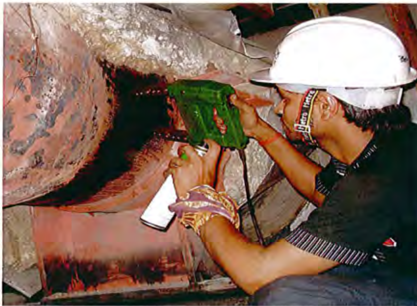
The view of MPI on MS line weld joint near strainer Ground floor.
