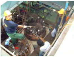
Heating with Burner
