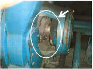
Photo-18: A-Vacuumpump grand seal (uncoupling side)
