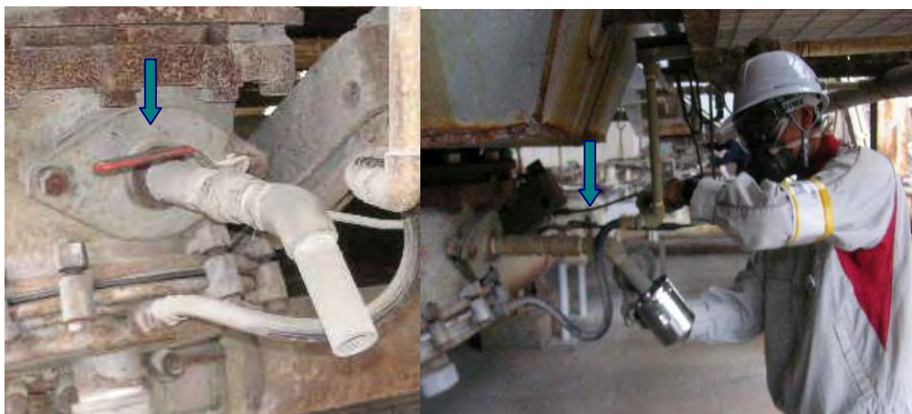
Fig. 6.13-2 Fly Ash Extraction Valve for Sampling
