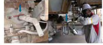
Fig. 6.13-2 Fly Ash Extraction Valve for Sampling
