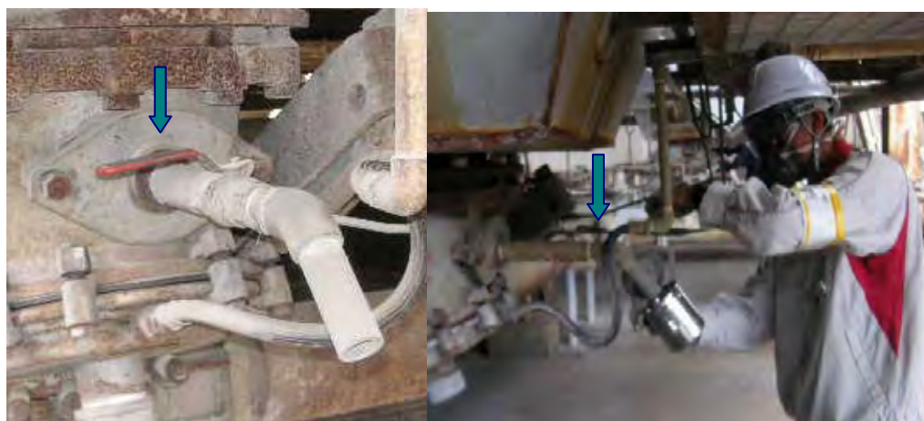
Fig. 6.13-2 Fly Ash Extraction Valve for Sampling
