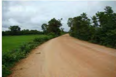
Good Gravel Section
