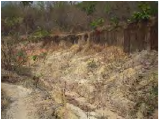
On-going large scale erosion around the bridge site.
