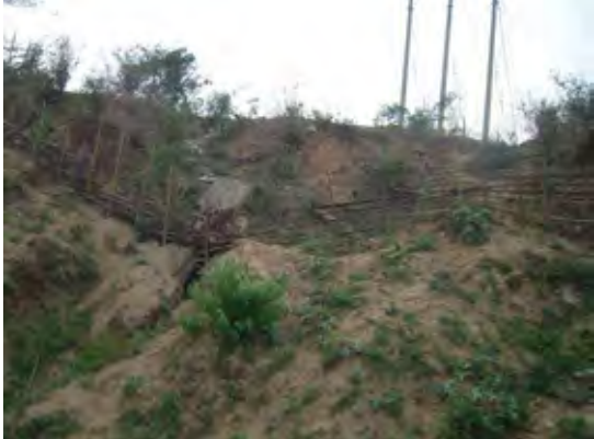
Small-scale landslide occurred on the riverbank slope.
