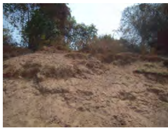
Unprotected River Bank (Eastside)
