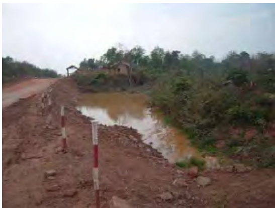
Roadside Inundation at bridge construction site
