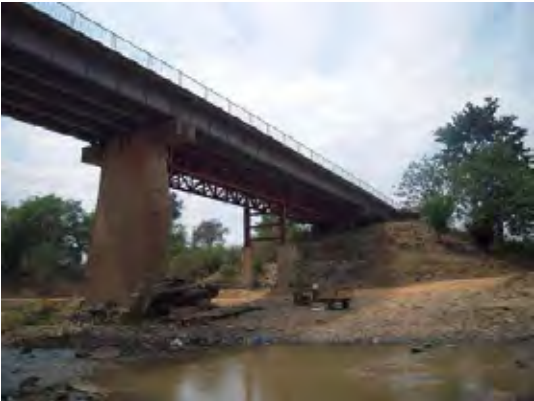
Debris, wood trapped at the bridge pier
