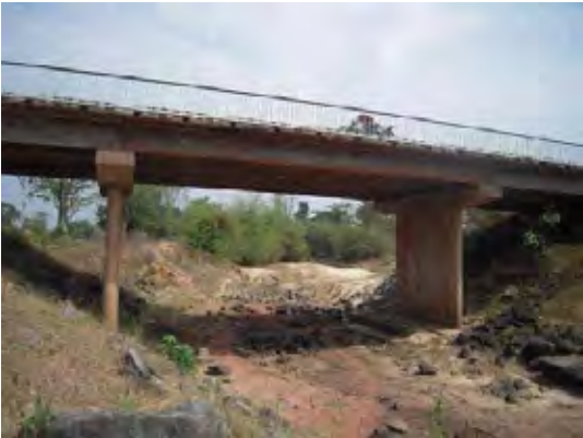
Dried up river bed condition of small-middle class bridge. Several large boulders exist
