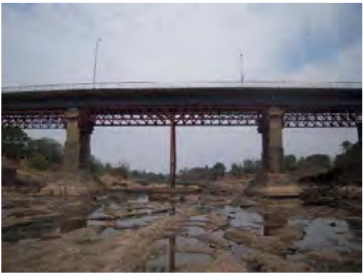
Low water level-river bed condition. Many traces of scouring are observed across entire river bed.
