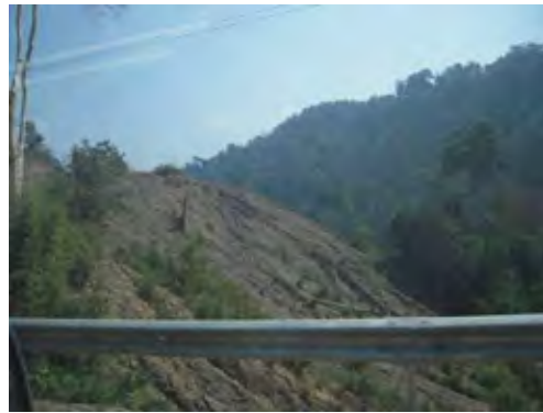
Mountain Cutting without proper vegetation cover (Route 18B, Attapeu Province). Large-scale erosion is on-going.
