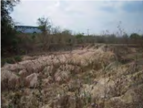
Erosion/gulleys found along Route 9 (Savannakhet Province)
