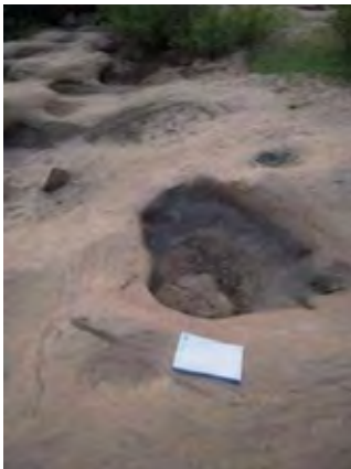
Scouring observed at Sebanhiang River, Savannakhet Province
