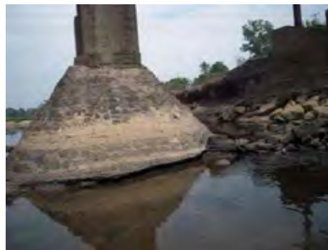
Scouring observed at Bridge Pier, Route 9, Savannakhet Province
