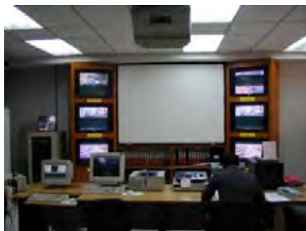
Traffic Control Center
