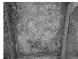
Source: JICA team Figure 3.4.15 Rust pit cover
