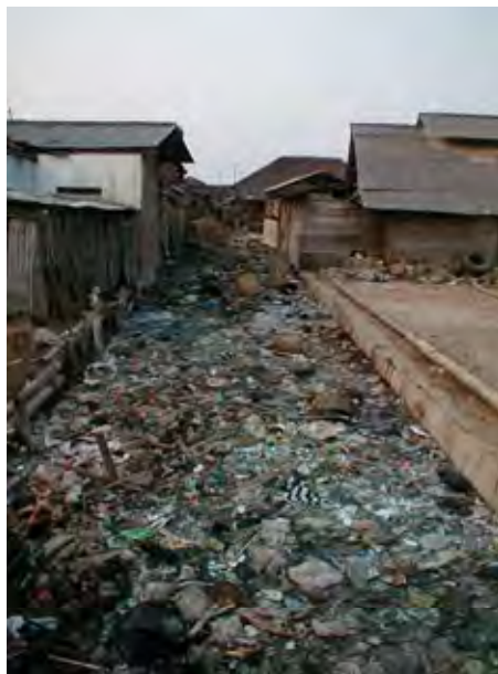
Fig. 4.2.7 Clogging of city main drain (from Appendix A)
