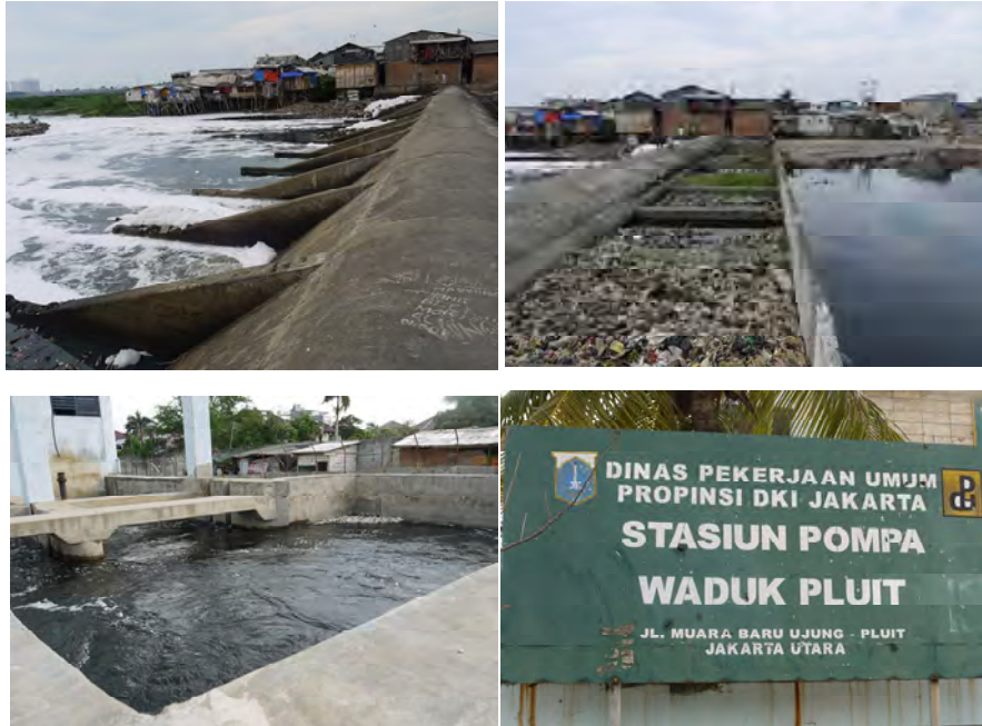
Fig. 4.2.15 South entrance barrage (weir) of the Pluit Lake (top) and the pump station in northern mouth of the lake (bottom-left)
