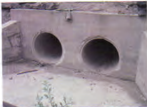
Culvert 9: No problem with its structure. Maintenance of road surface is necessary.
