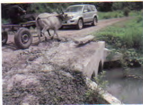
Culvert 7: No problem with its structure. Maintenance of road surface is necessary.
