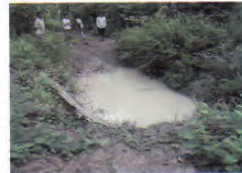
Culvert 4: The bent road next to the culvert needs to be repaired.
