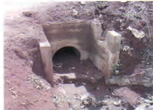
Culvert 2 installed at the same road as culvert 1: Needs clearance of mud.
