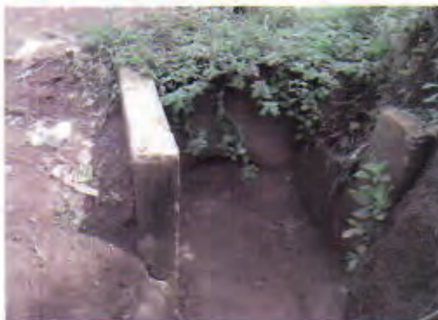
Culvert 3 installed at a road in the district capital: Needs clearance of mud. Initially, a master plan of drainage system for the entire city and periodical maintenance is necessary because this point is in the lowest level of the surrounding area.
