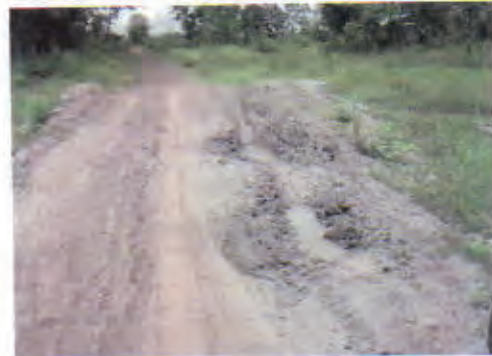
Culvert 8: No problem with its structure. Maintenance of road surface is necessary.
