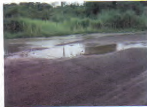
The road has no problem. However, to avoid crucial damage on the road by water flow from streams nearby, construction of ditch/ channel is necessary.
