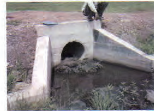
Culvert 4: No problem. Photo shows a local irrigation way to control water flow by installing mud and grass.
