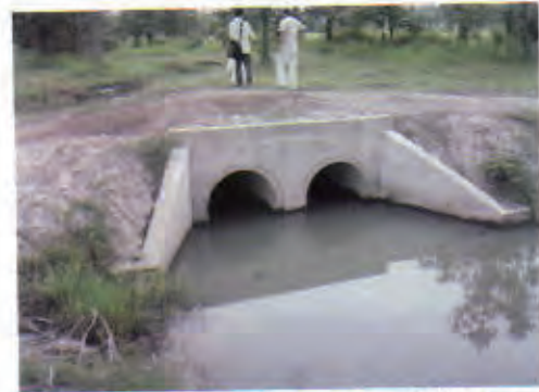
Culvert 6: No problem with its structure. Maintenance of road surface is necessary.
