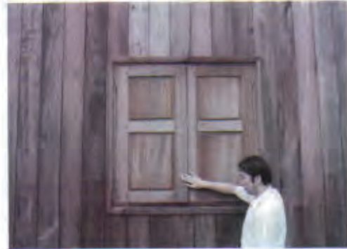
This window has a problem for opening, which will be solved by changing the installation point to upward or cutting the window bottom to adjust its frame size.
