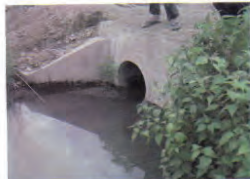
An example of the culvert installation project financed by Commune Fund: Its conduit size seems to be small for this location.
