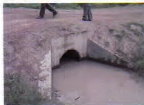
Culvert 2: No problem with its structure. Maintenance of road surface is necessary.
