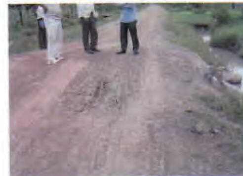
Culvert 2: The road surface is bent due to heavy traffic.
