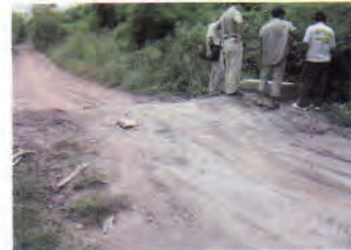
Culvert 3 at a road leading to Vietnam: There are damage and exposure of concrete structure due to heavy trucks.
