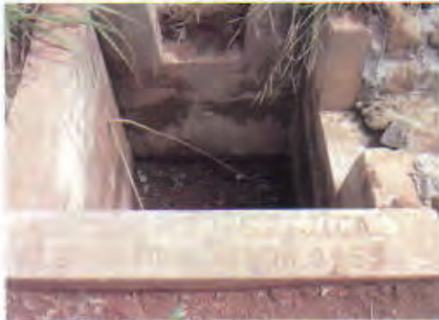
Culvert 1 installed at a road in the district capital: Needs clearance of mud.
