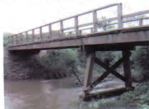
The bridge has no problem. However, for sustainable use, maintenance of bridge including clearance of obstacles to flow in the river is necessary.
