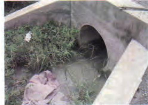
Culvert 1: This place looks like a garbage dump due to lack of public morals.
