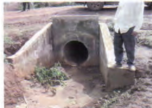
Culvert 4: No problem with its structure. However, the level of drainage is higher than the conduit level due to coverings such as mud and garbage, which may cause overflow or backwater and then heavy damage in this area afterwards.
