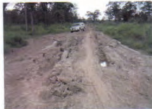
Culvert 9: Maintenance of road surface is necessary. The commune is planning to repair by Commune Fund.
