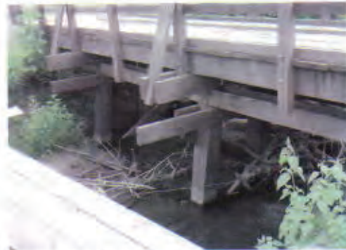
No problem with the bridge. Maintenance of road surface, canal and limit of weight are necessary for sustainable use
