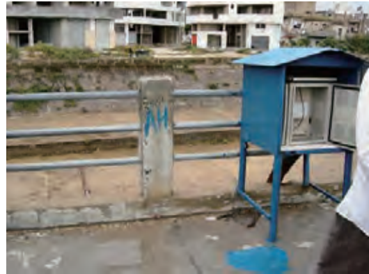
[WRIC015] "Al Gmka River" Water Level Station Equipment was moved from the bridge to approx. 100m upstream to avoid tidal effect.
