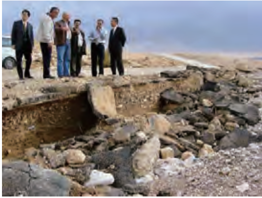
[WRIC012] River was flooded caused by discharge from upstream dam few days ago and road was severely damaged by bank erosion.
