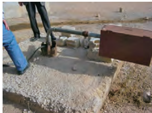
[WRIC034] "Safa" Pumping Well Candidate meteorological equipment and groundwater level gauge installation site for Badya Basin, however, this well is used for pumping and seemed to be not suitable for groundwater level observation.
