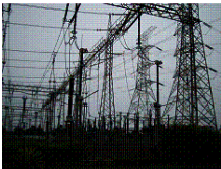
Gambar 3.6-18 500kV transmission facility
