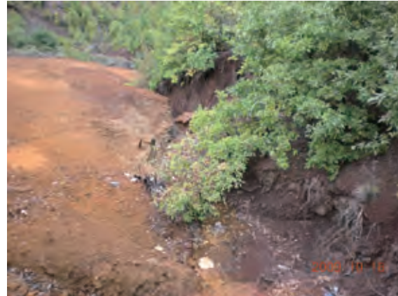
Photograph 5.6.18 Deep erosion on the right
