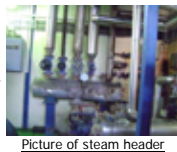
Picture of steam header
