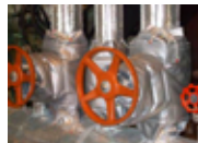
Valve insulation by insulation jacket
