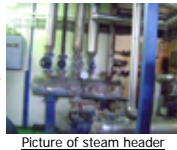
Picture of steam header
