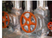
Valve insulation by insulation jacket
