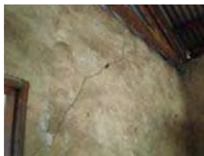
Many cracks on the wall
