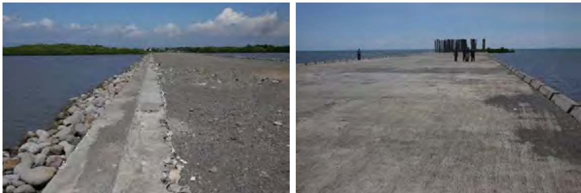
Fig. 4.2-10 Current view of the construction site of PPN Untia (Source: Survey team)
