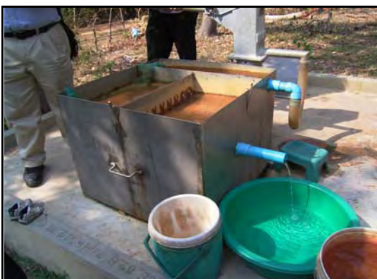
Photo 4-5 Iron removal unit for groundwater.
