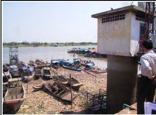
Photo 4-1 intake facility of provincial capital water. intake pipe is induced beneath the derrick and pump is installed in the concrete room. Poor raw water quality.
