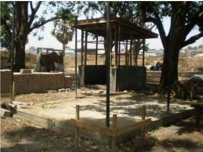
Generator Shed & Fuel Storage
