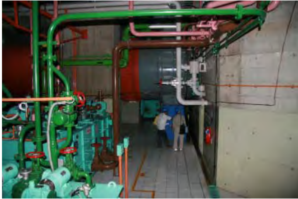
Inlet Valve Floor
