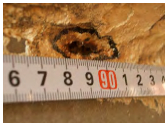
Pitting Corrosion at Outlet Side
