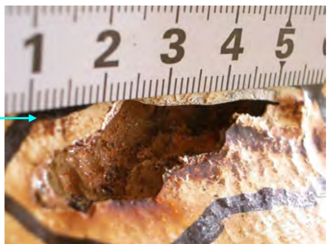
Detail of Pitting Corrosion)
