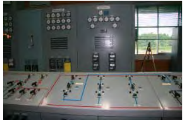
Control Desk for Operation
