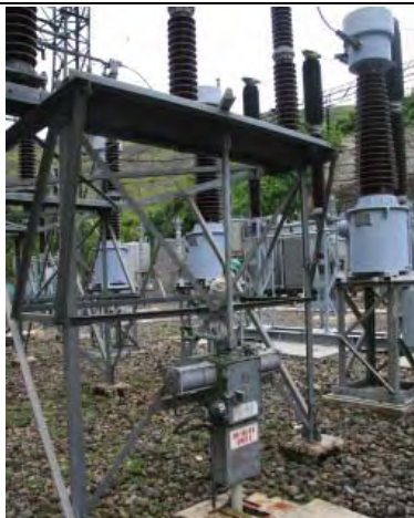
154kV Disconnecting Switch
