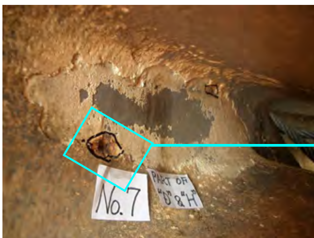
Pitting Corrosion and Cloudy Cavitation at Outlet Side
