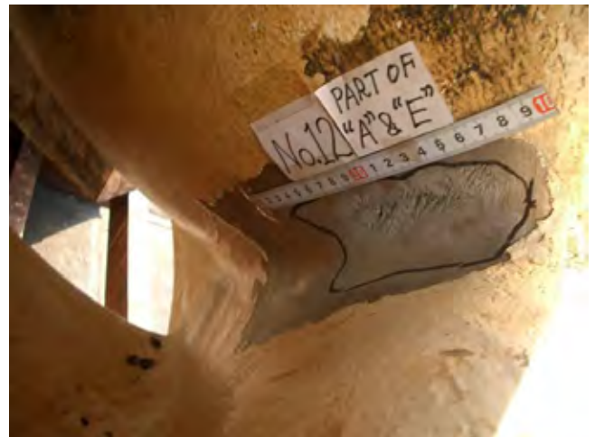
Cavitation and Paint Peeled Area at Inlet Side
