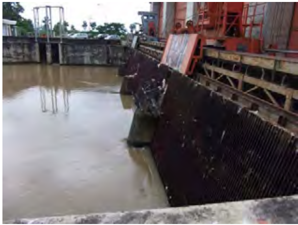
Power Intake - Trashrack
