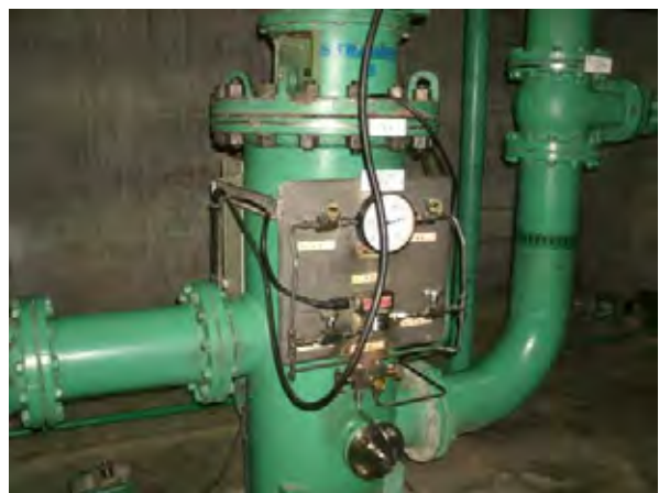
Strainer for Cooling Water System
