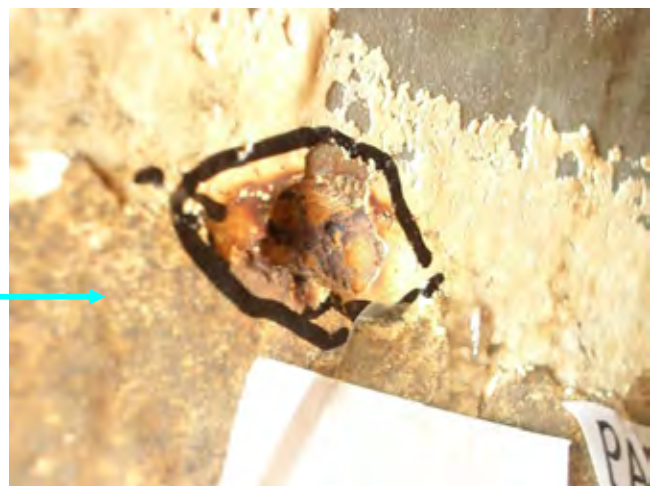
Pitting Corrosion at Outlet Side
