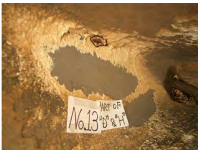
Pitting Corrosion and Cloudy Cavitation at Outlet Side
