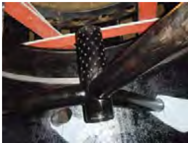
Aeration Pipe (Below Runner)
