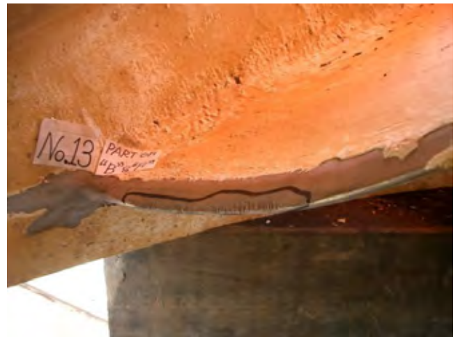
Cavitation and Paint Peeled Area at Outlet Side
