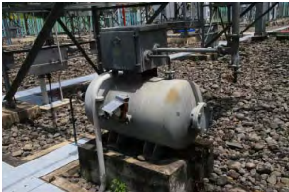
154kV Disconnecting Switch Air drive
