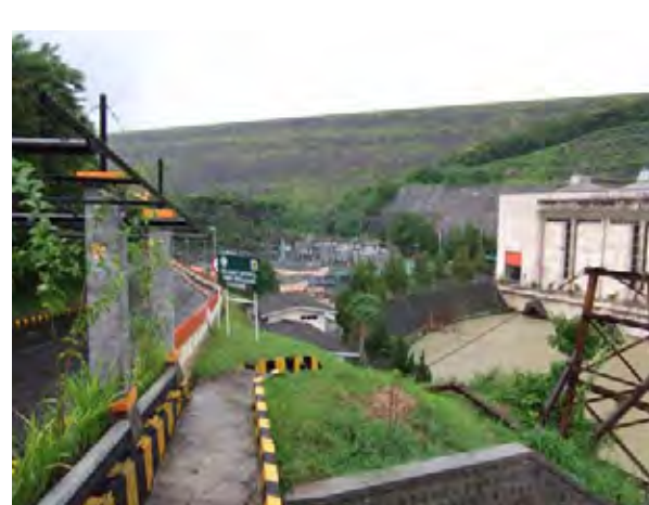
Power Station - Outdoor Switch-yard
