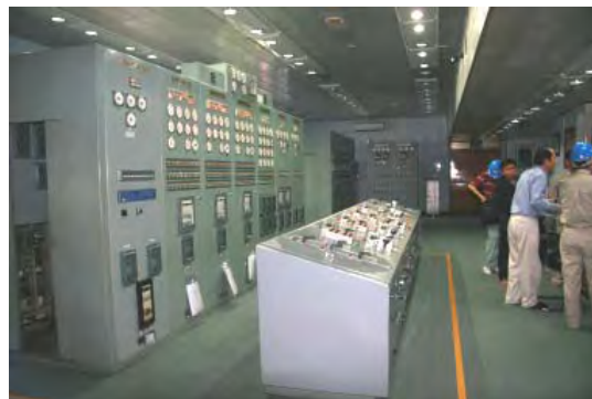
Control Panel and Operation Desk
